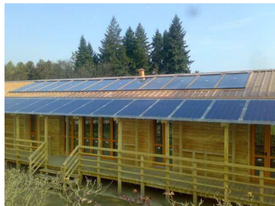
Fig. 1: Picture of the new building with integrated solar thermal (up) and photovoltaic collectors (bottom)
